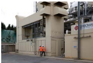
Photo: Solar Turbines Outside Paris, France, a Mars 100 gas turbine transforms landfill gas into electricity.
